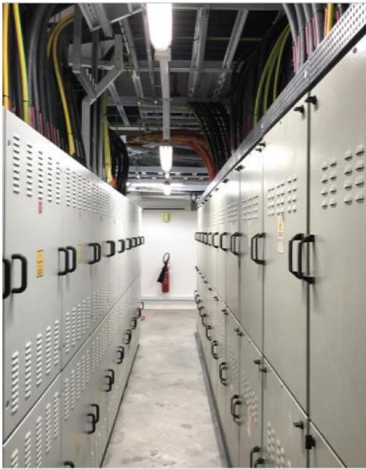
Fig 1. Cooled Space area East Wing LV Switch Room 1
