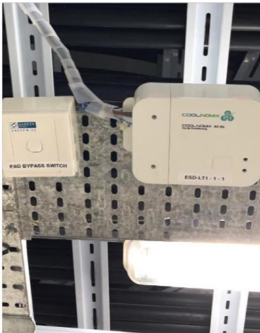
Fig 3. COOLNOMIX unit connected to FCU-E-LT1-1-1
